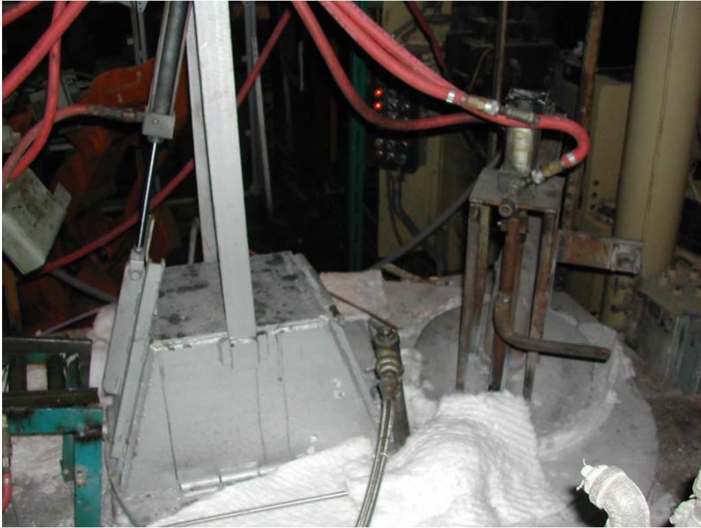
Figure 1-1. Die Casting Machine Crucible at Lunt Manufacturing
